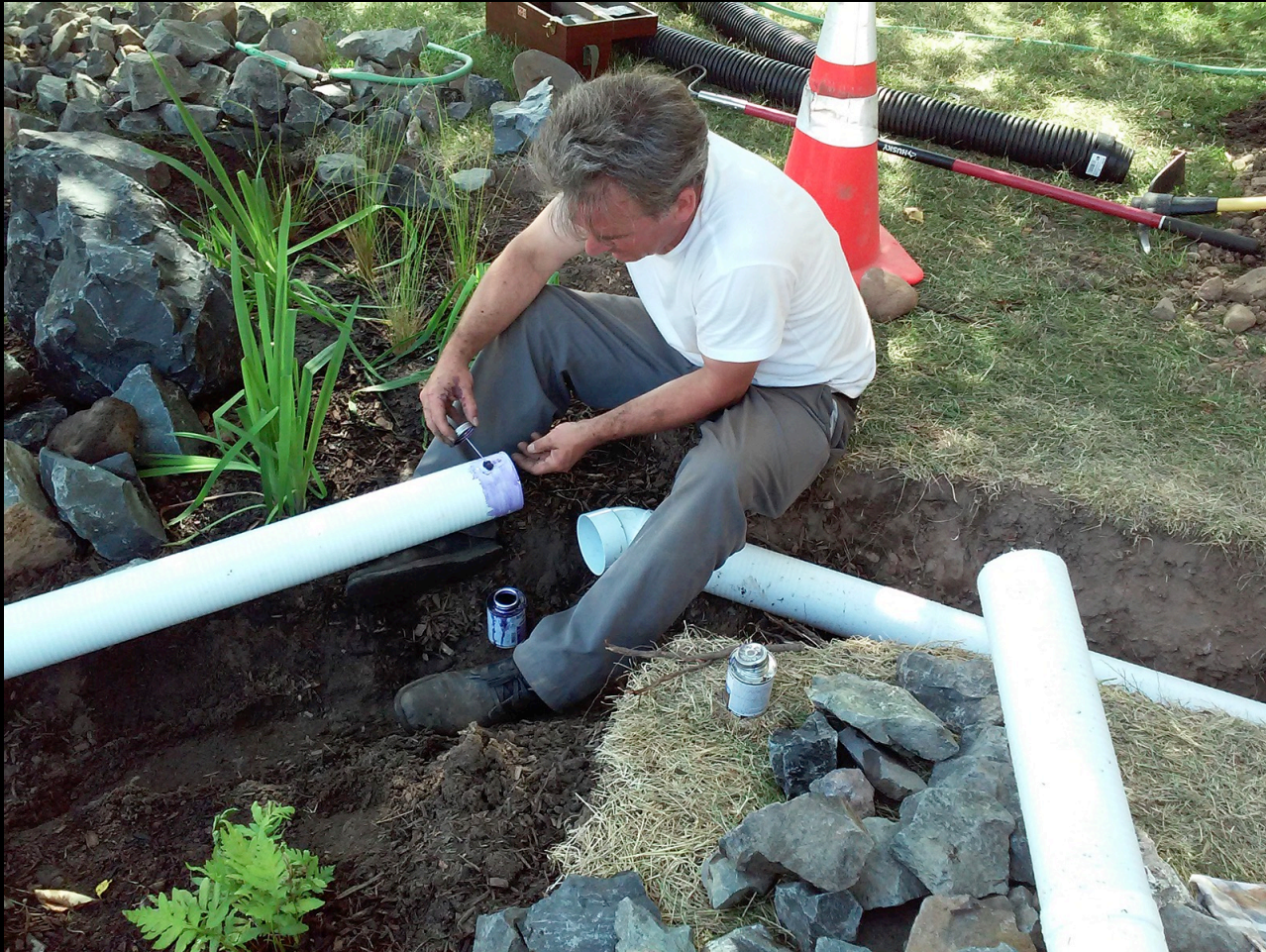
Stormwater from the downspout is piped into the garden through the trench.
