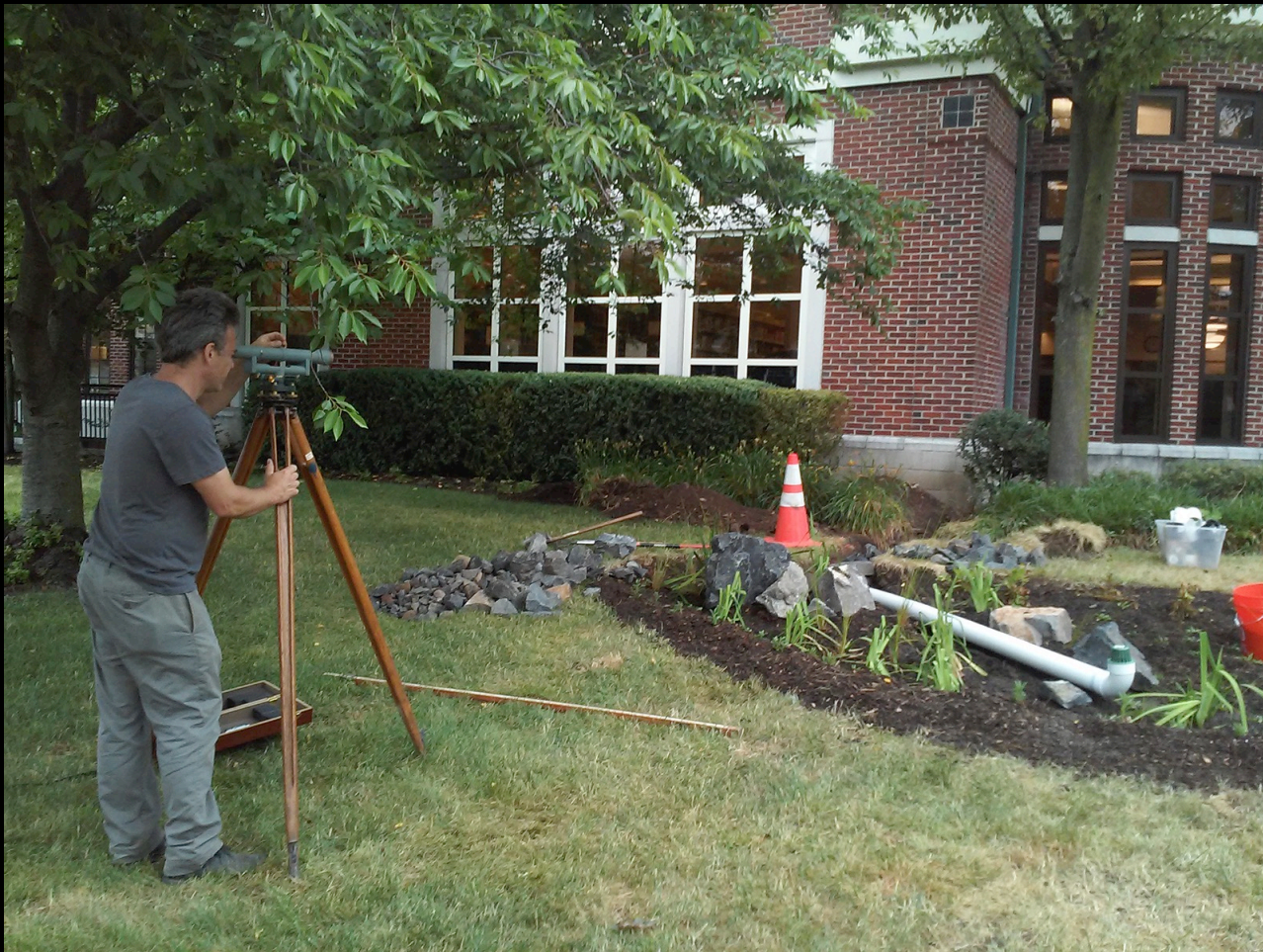
Checking the level to be sure water flows in the right direction.
